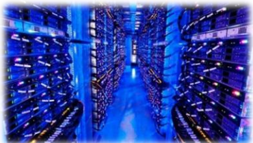
Servers and HPCs
